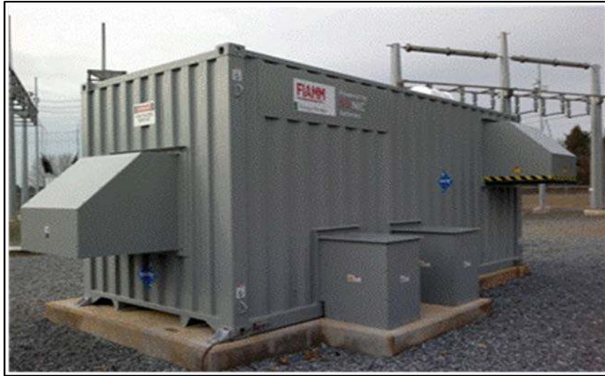
Figure 39. FIAMM 222-kWh System Site at the Duke Energy Rankin Substation
