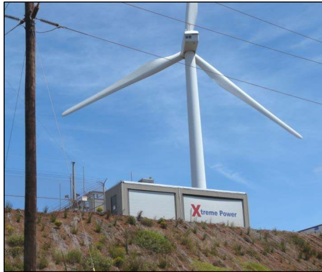
Figure 72. 1.5-MW/1-MWh Advanced Lead-acid Dry Cell Systems by Xtreme Power in a Maui Wind Farm (Source: Xtreme Power)
