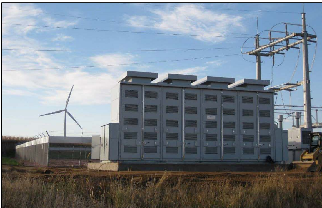
Figure 34. Xcel Battery Supplementing Wind Turbines, Lucerne, MN
