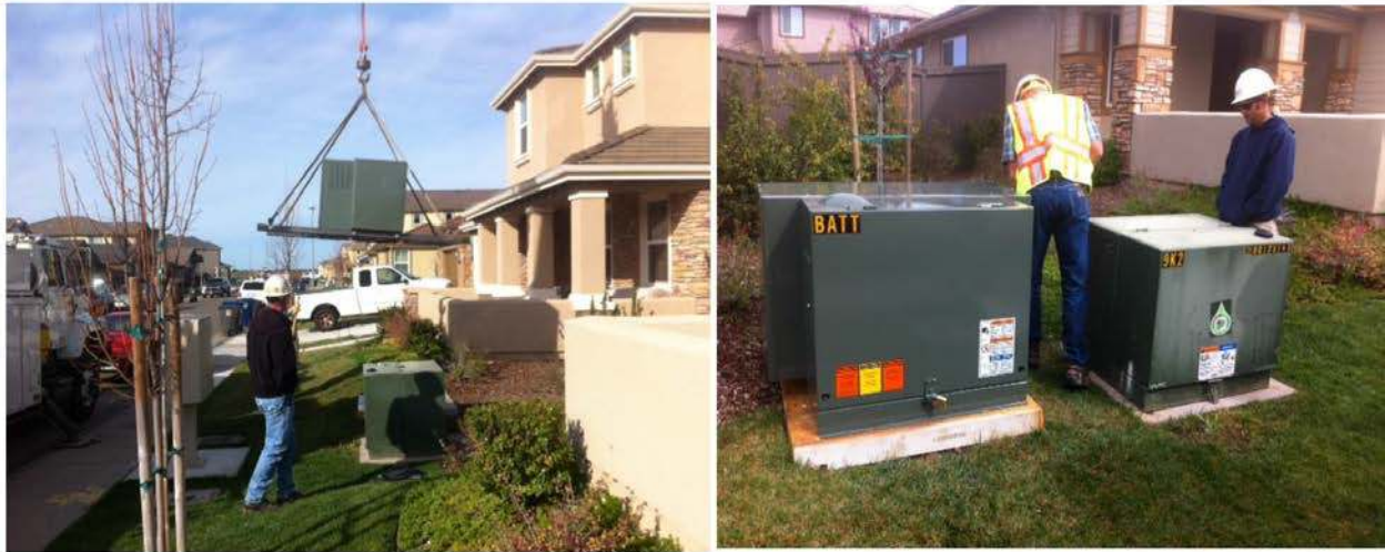
Figure 99. A 30-kW/34-kWh Distributed Energy Storage Unit (Being Installed and Inspected at the Sacramento Municipal Utility District's Anatolia SolarSmart Homes Development. Suppliers are SAFT, Grid Point, and Power Hub)
