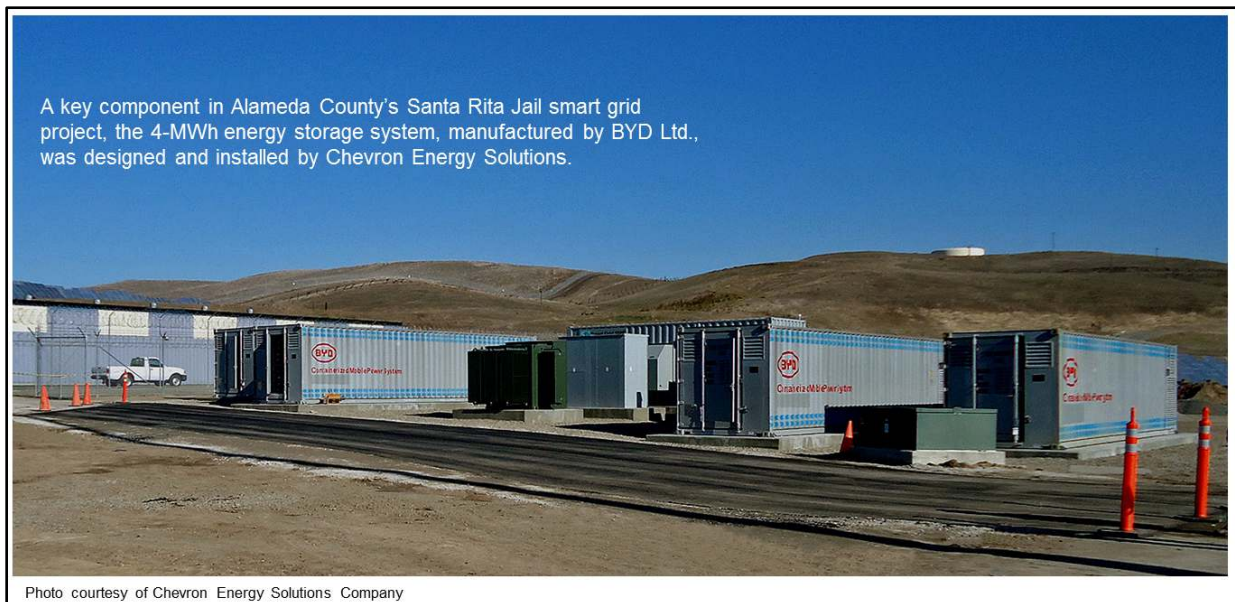
Figure 98. A 2-MW/4-MWh Li-ion Energy Storage System
