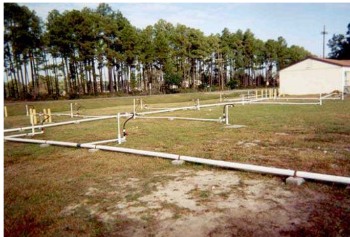
Figure B-1. MPE Extraction Wells
