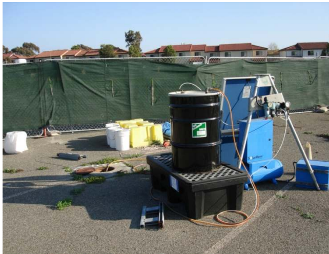
Figure A-1. Solar Powered Skimming System for LNAPL Recovery (see blue equipment)
