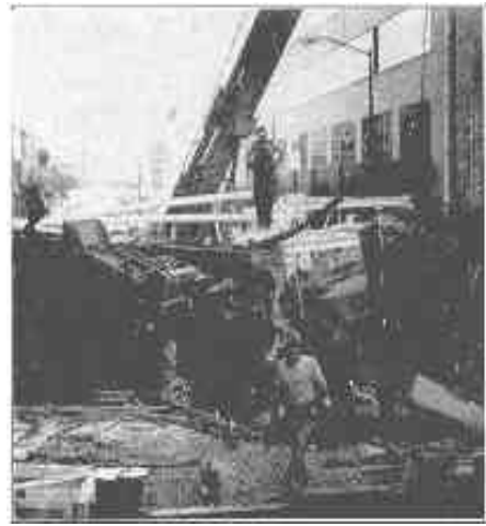
TOWER CRANE COLLAPSE (CLEANING UP DEBRIS)
