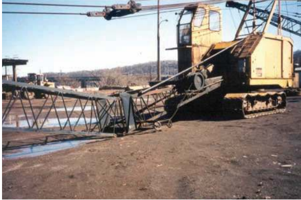
Figure 7. Boom collapse during crane disassembly.
