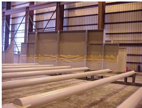
Figure 18 Photo showing painted members in a fabrication shop, note the masked area is for prime coat only
