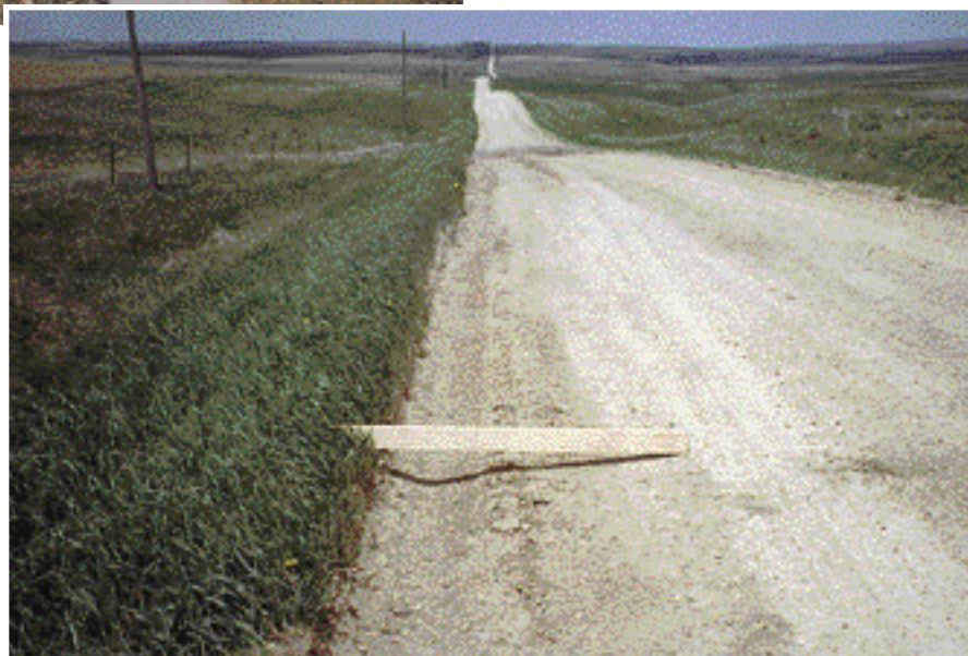
Secondary ditch over six inches deep.
