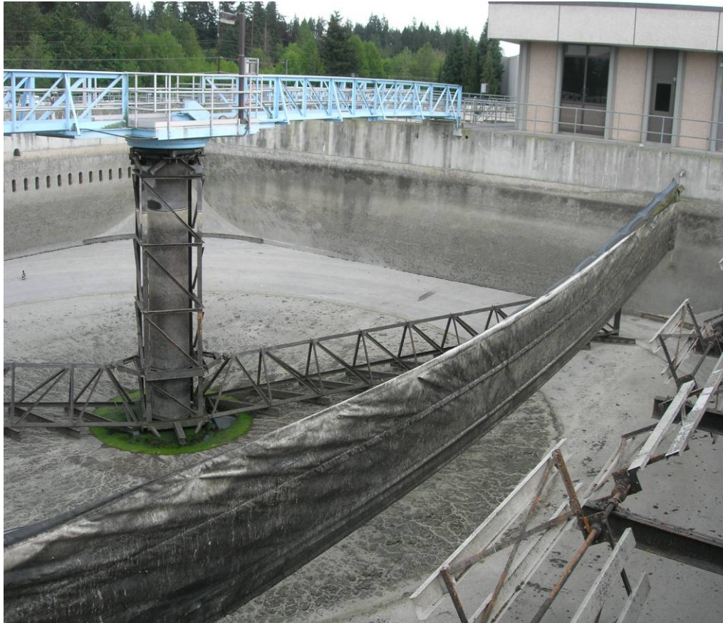
Empty tertiary clarifier at Clean Water Services, Durham AWWTP
