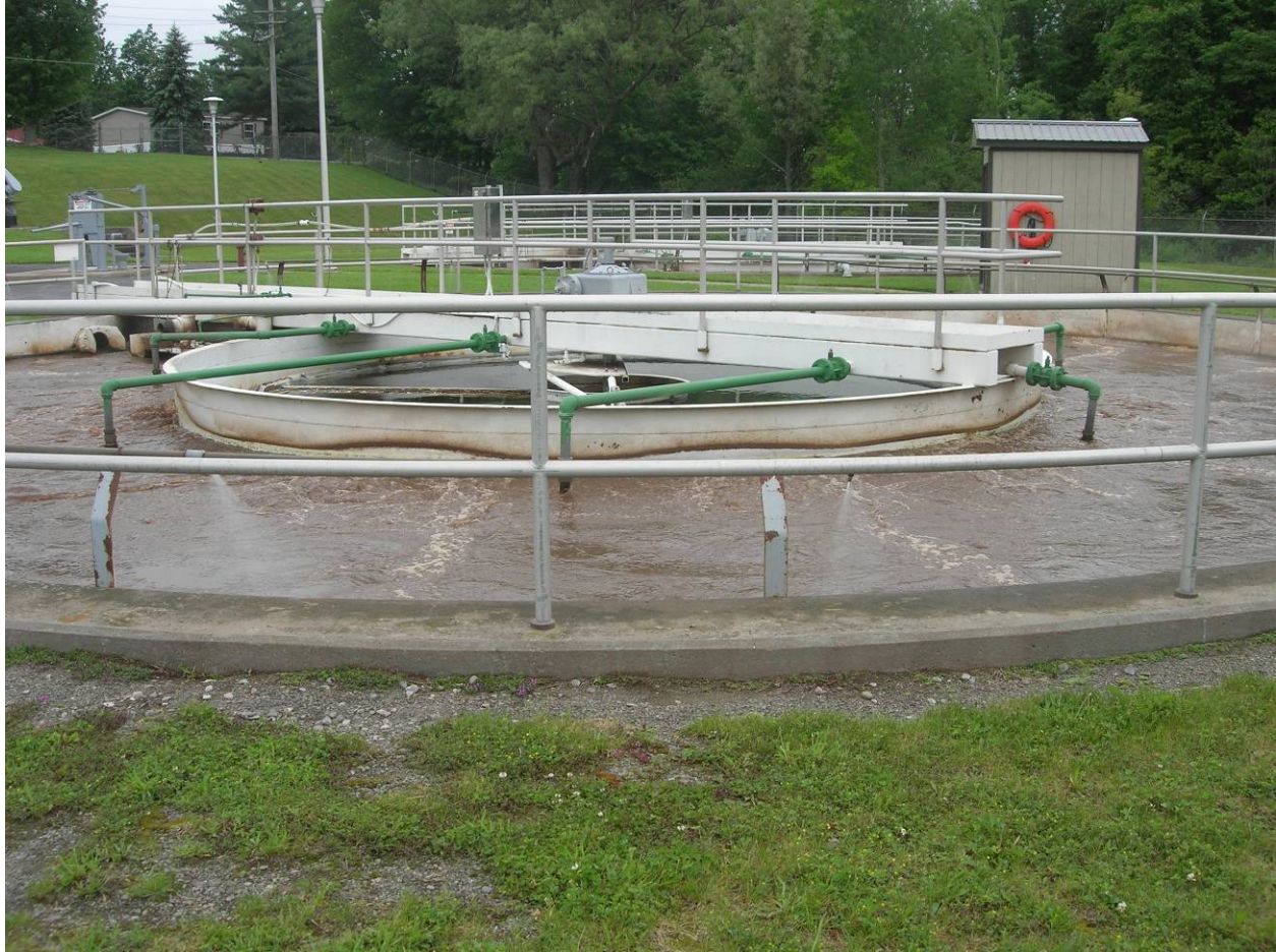
Combined aeration basin and clarifier (in center of unit) at Stamford WWTP
