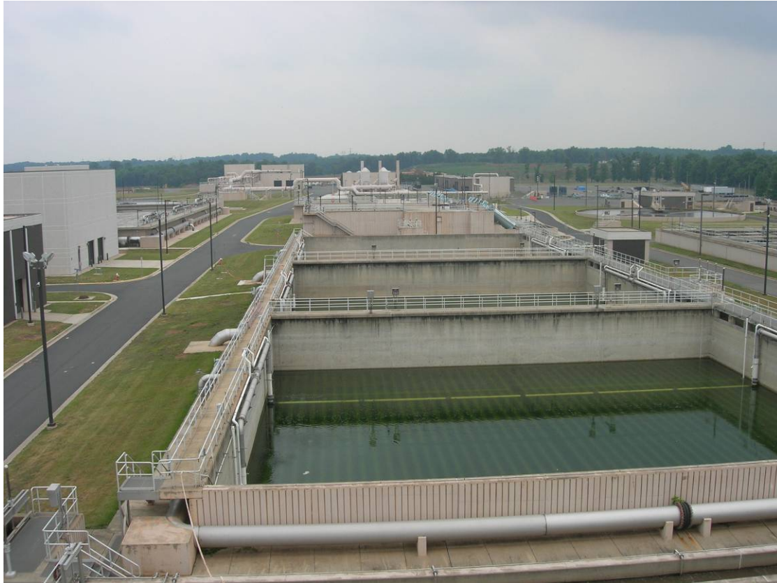
UOSA Water Reclamation Facility (WRF) – in the forefront are fine bubble diffuse aeration basins constructed during the plant expansion to 27 mgd which are off-line in this picture.
