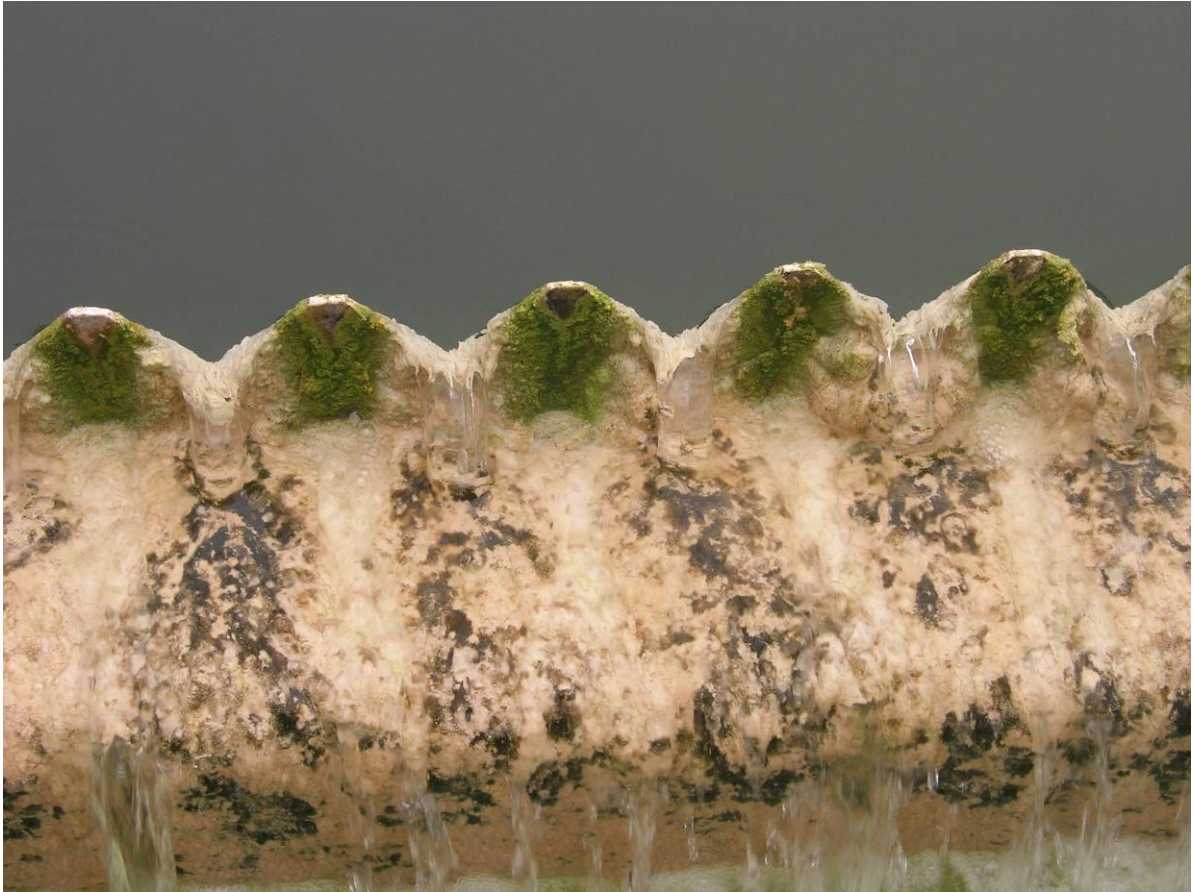
Lime scaling on chemical clarifier weirs at the UOSA WRF
