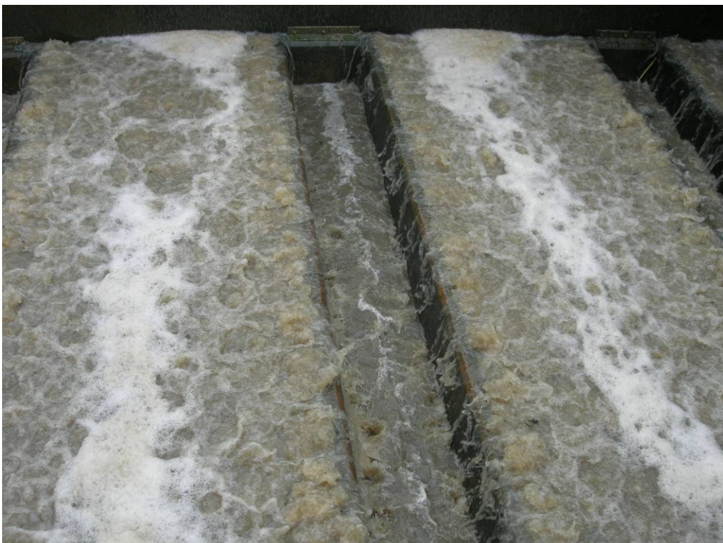
Bed filter undergoing backwash at Alexandria AWWTP
