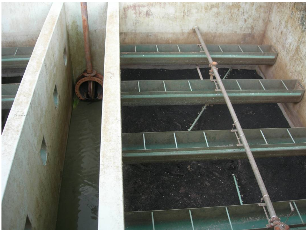
Empty gravity flow bed filter at Clean Water Services, Durham AWWTP
