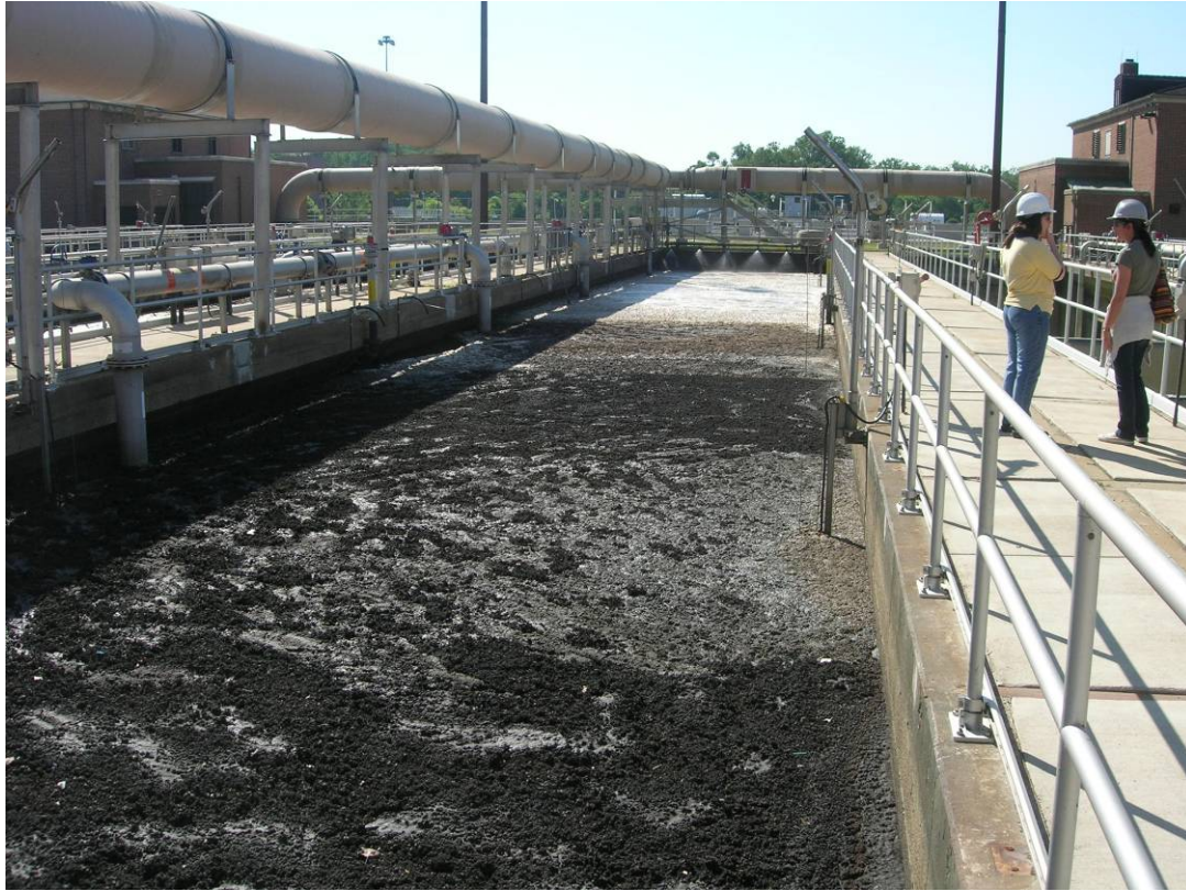
Wastewater contact basin in operation at Noman Cole PCP
