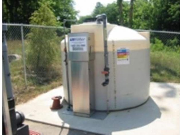
Figure 7. Nitrate Storage and Delivery System
