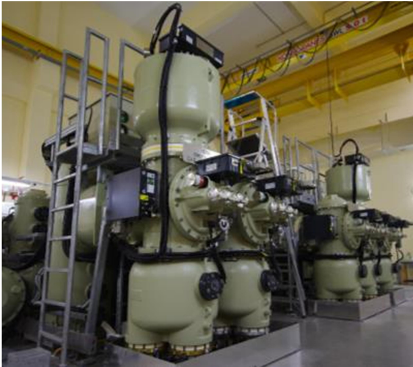
Figure 1. Ladders and platforms in GIS
