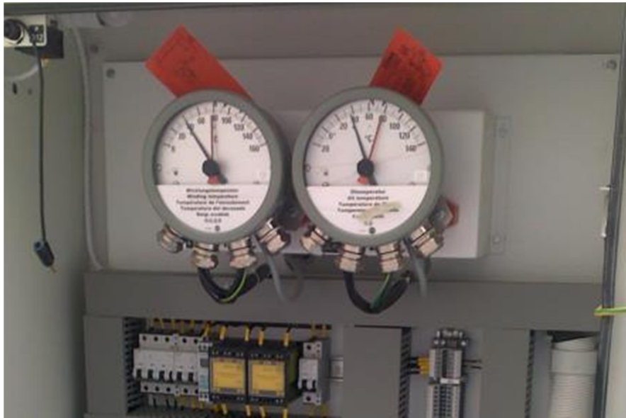
Figure 2. Gas density monitoring indicator
