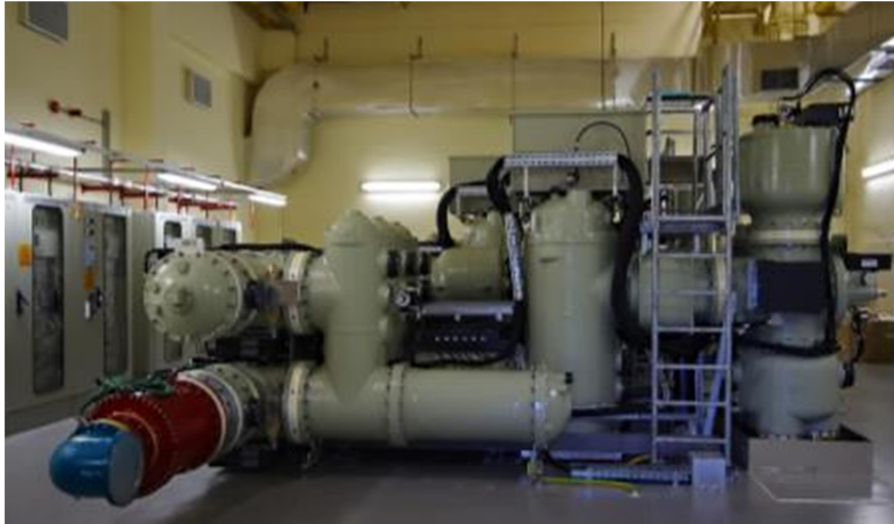
Figure 7. SF6 gas to cable connections
