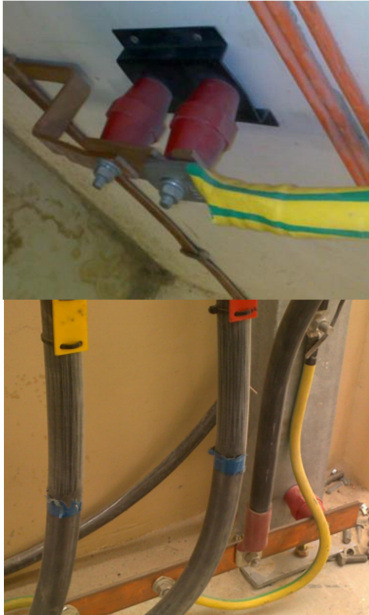
Figure 5. Ground/earth connection of GIS using bolts or a steel bar in the floor (a) Bolted GIS fixing with grounding connection (b) Steel bar is the floor including grounding connection
