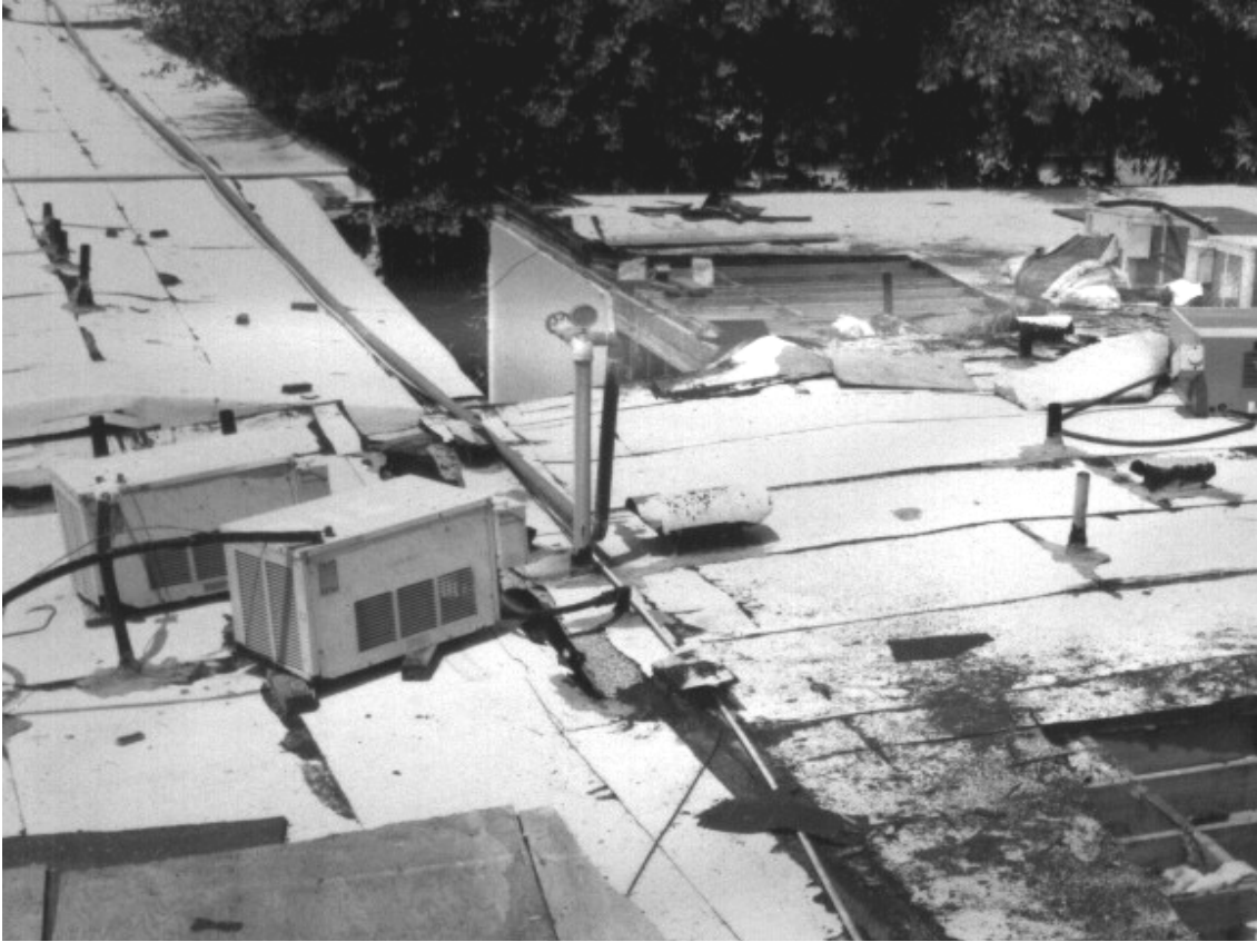
Figure 2-12 Roof-level damage to building with a T-shaped plan. The damage at the roof corner (right-hand side) is due to stress concentrations where the wings of the building connect.
