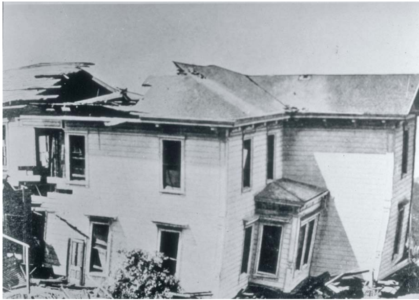
Figure 1-6 A house damaged due to fault movement. The fault passed under this house near Wright's Station, on the Southern Pacific Railroad, in Santa Cruz County, California. The house was severed by fault movement during the earthquake. Photo credit: R.L. Humphrey, U.S. Geological Survey.
