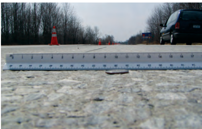
Figure 7.8 Diamond ground surface after years of service (photo courtesy of The Transtec Group)
