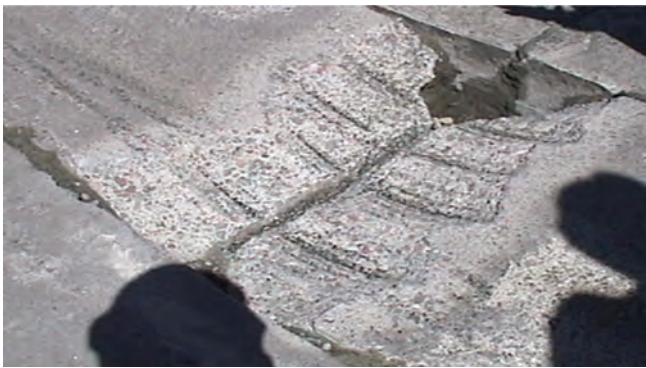
Figure 7.4 Damaged material has been milled out in a partial-depth repair (photo courtesy of Dale Harrington, Snyder and Associates)
