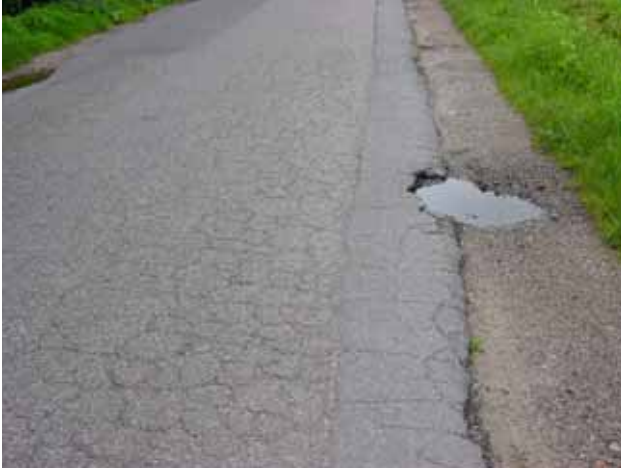
Figure 3: Cracking observed on a narrow polder road in the Netherlands.
