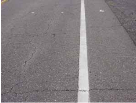
Figure 5: Low temperature associated block cracking observed on a highway in Minnesota.
