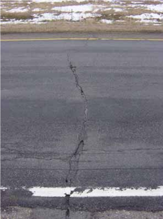
Figure 4: Low temperature cracking observed on a highway in Minnesota.
