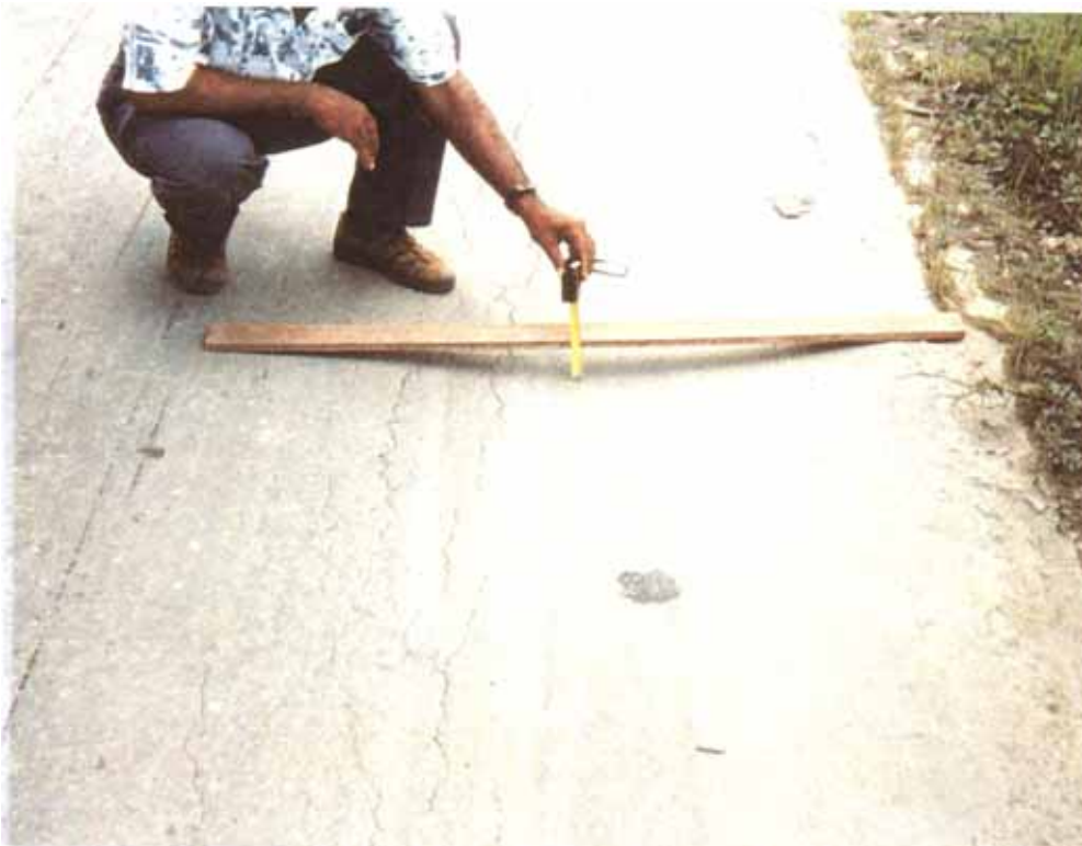
Figure 98: Excessive pavement deformation due to deformation of the unbound base and/or sub-base layer.
