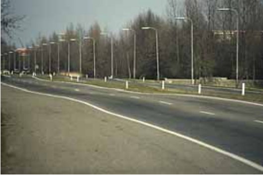
Figure 10: Longitudinal deformations due to settlements.
