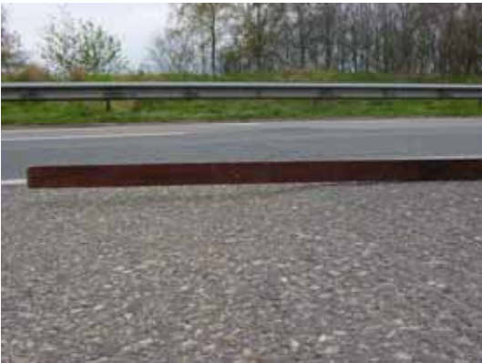
Figure 12: Unevenness due to "buckling" of the base made of blast furnace slag.
