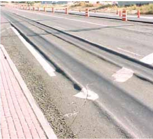
Figure 11: Rutting in an asphalt pavement.
