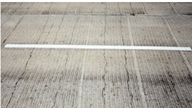
Fig. 6-17. Shrinkage cracks, such as shown on this bridge deck, can be reduced with the use of good concreting practices and shrinkage reducing admixtures. (69883)
