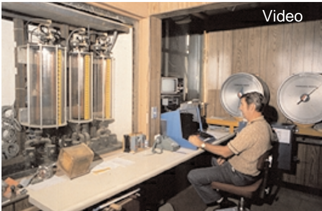
Fig. 6-20. Liquid admixture dispenser at a ready mix plant provides accurate volumetric measurement of admixtures. (44220)
