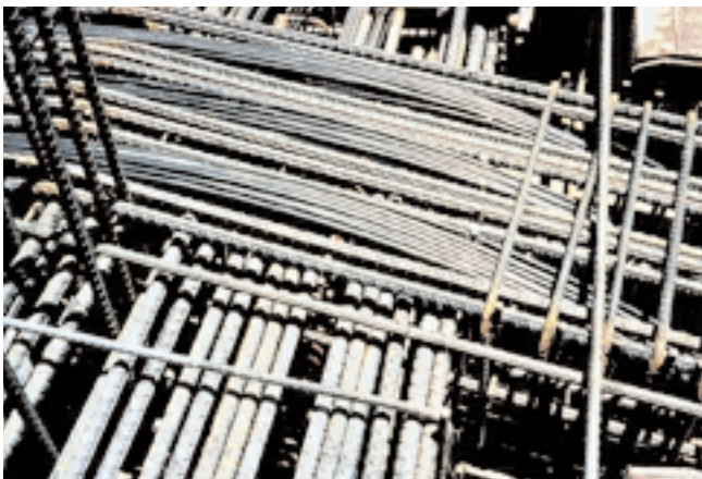
Fig. 6-9. Flowable concrete with a high slump (top) is easily placed (middle), even in areas of heavy reinforcing steel congestion (bottom). (47343, 69900, 47344)
