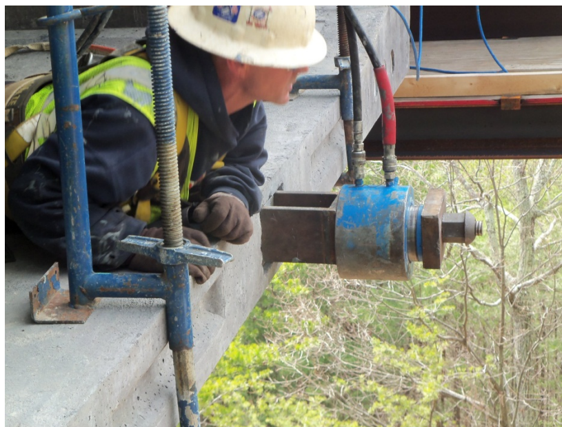
Figure 1.36 - Stressing Temporary Bar in Bottom Slab of the Foothills Parkway Bridge No. 2
