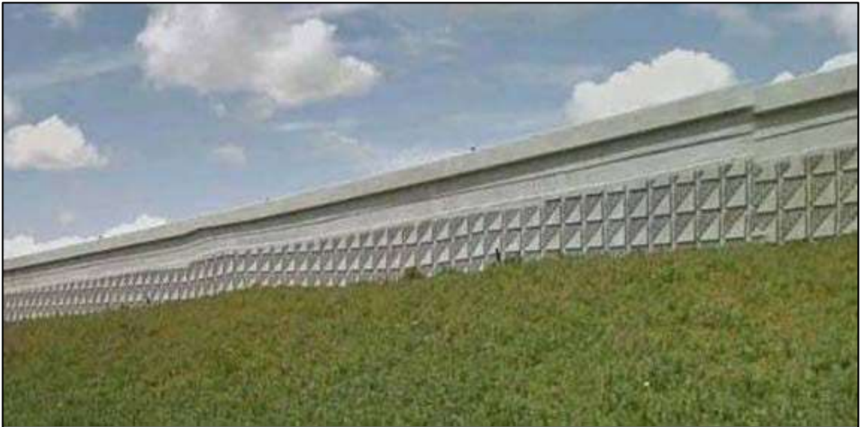
The staggered appearance and misaligned pattern of this wall structure are the result of inadequate coordination of the aesthetic design, wall design, and construction methods.
