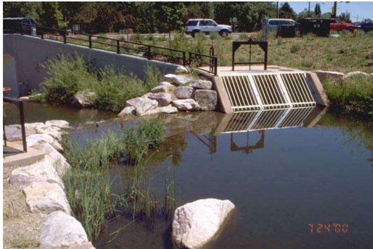
Photograph CU-4—Public safety features such as the rack at the entrance to an irrigation ditch and the railing on the wingwalls must be considered.
