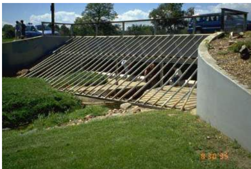
Photograph CU-1—Public safety considerations for long culverts should be accounted for with culvert designs such as with this collapsible trash rack at a park-like location.
